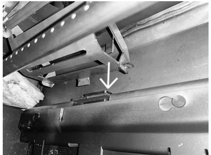
Figure 9: Remove Flue Gas Agitator
